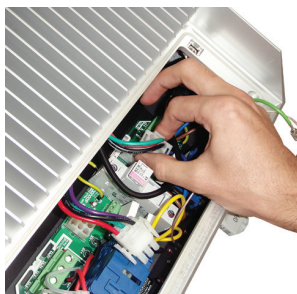
Disconnecting Inverter Module Plugs
